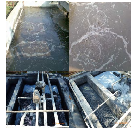
Oxygenation in the aeration basin
